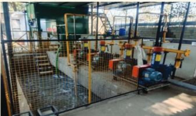
ETP PLANT WITH MBBR TECHNOLOGY
